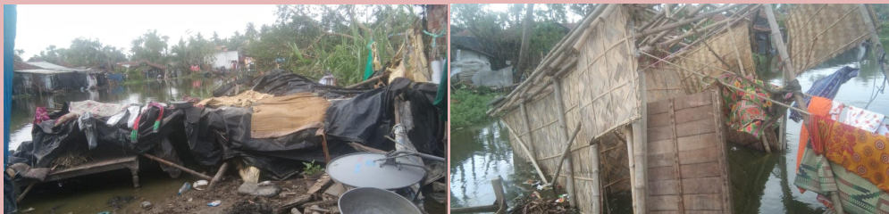
Damaged huts after Amphan Cyclone
